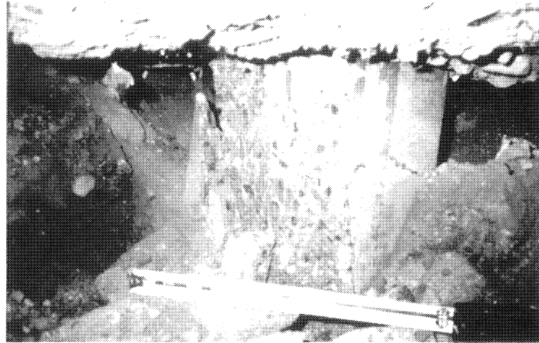
Fig. 5.23: Pile Damage at Los Virgenes Overcrossing
