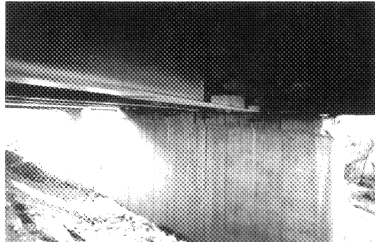
Fig. 5.21: Pier Wall at Southbound Span of Santa Clara River Bridge Looking South
