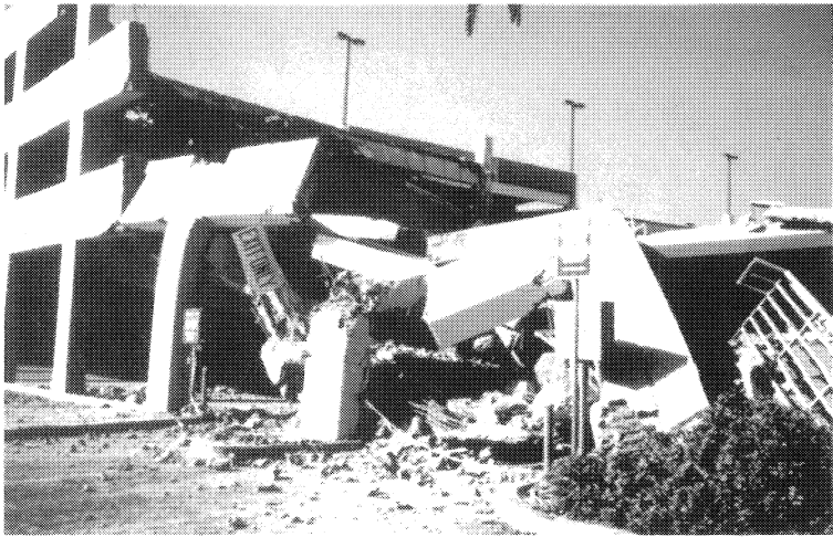
Fig. 6.7 Characteristic "Implosion" of Precast Parking Structure
