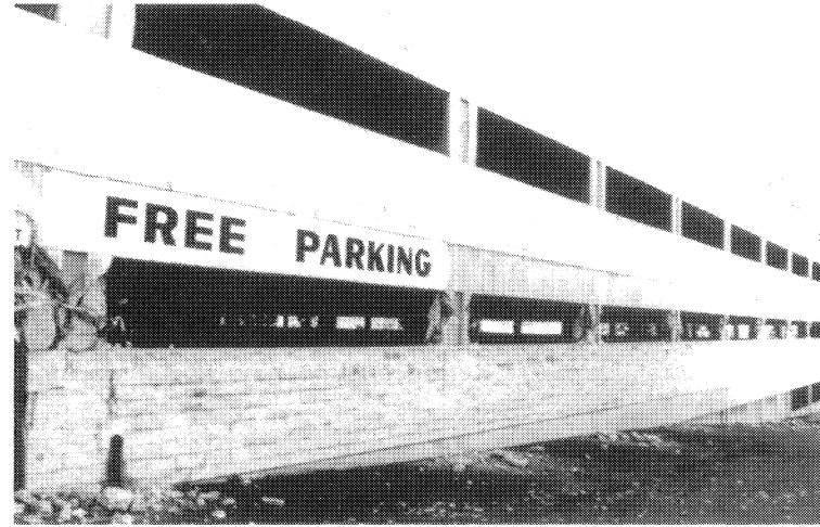
Fig. 6.8 Short Column Effect due to Partial Infill
