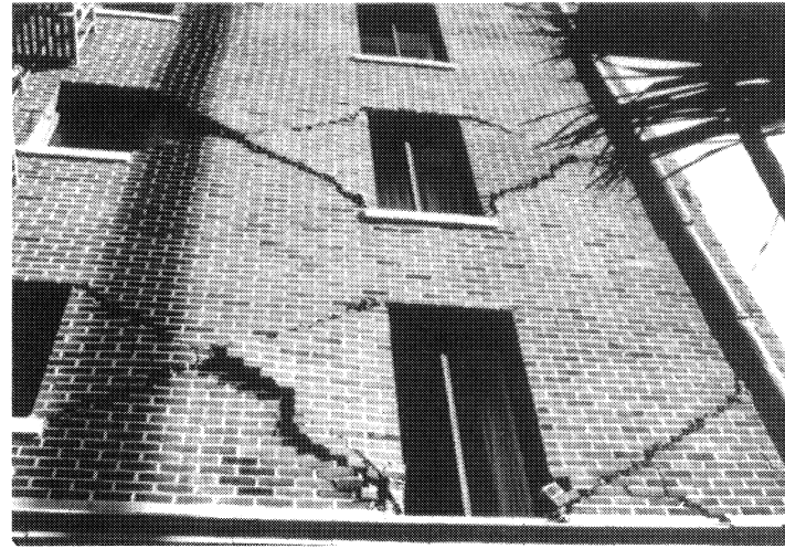
Fig. 6.14 Shear Cracking in Non-Bearing Masonry Wall
