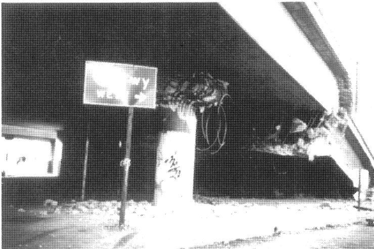
Fig. 5.16: Overview of La Cienega–Venice Undercrossing Collapse
