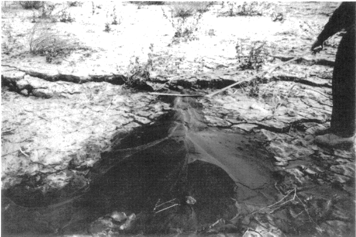
Fig. 4.5: Lateral spreading fissure and sand boil at dry lakebed behind Hansen Dam
