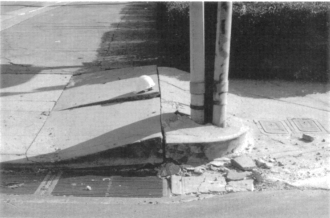
Fig. 4.8: Buckling of curb from lateral spreading, Northridge Hospital
