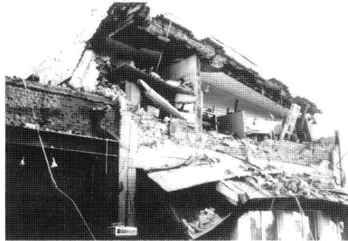
Fig. 6.16 Typical Shear and Out-of-Plane URM Failure
