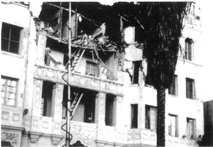
Fig. 6.15 Typical Shear and Out-of-Plane URM Failure
