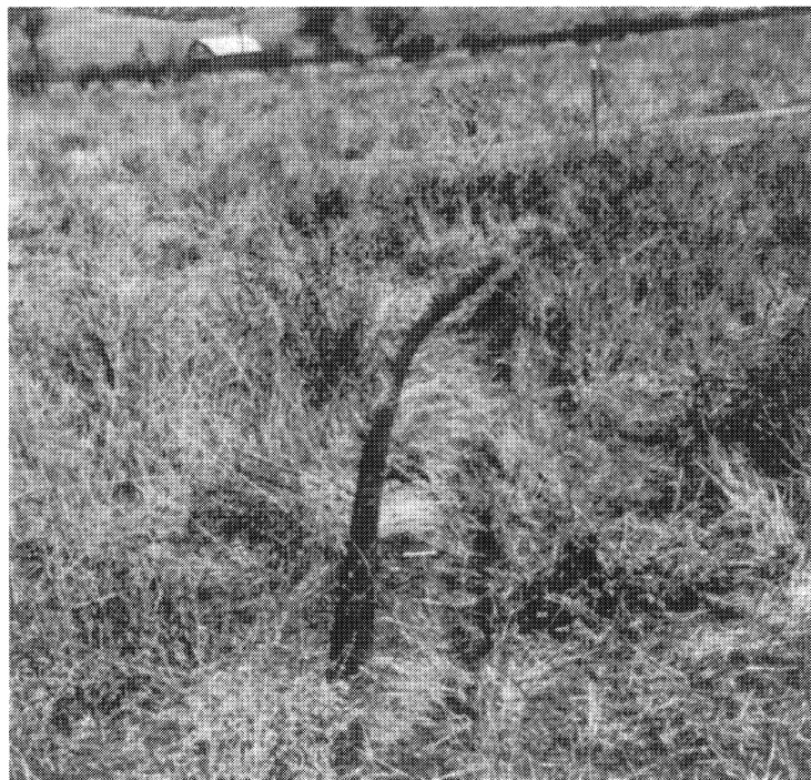
Fig. 4.3: Evidence of localized compression in Potrero Canyon. Note that originally straight pipe was pushed up and laterally; shortening across its length was 5 inches.
