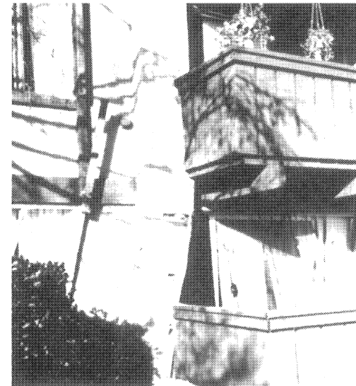
Fig. 6.20 Soft Story Collapse of Wood Apartment Building
