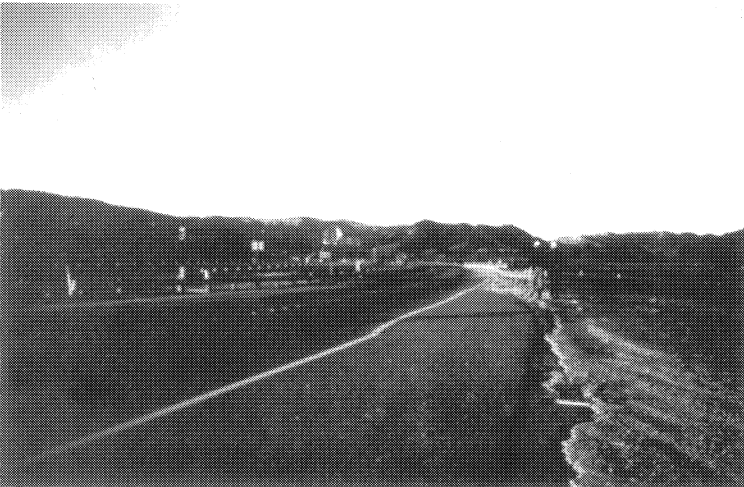
Fig. 5.24: Ground Cracks at East Approach of Interstate 5/Route 126 Separation
