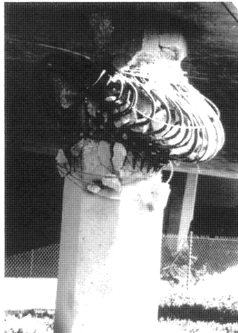
Fig. 5.9: Column Failure at Bent 2, Bull Creek Canyon Channel Bridge
