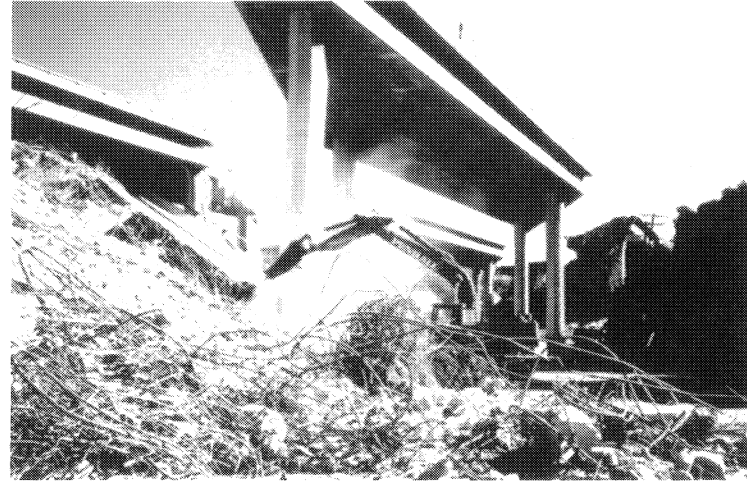
Fig. 5.19: Collapsed Spans at Gavin Canyon Undercrossing
