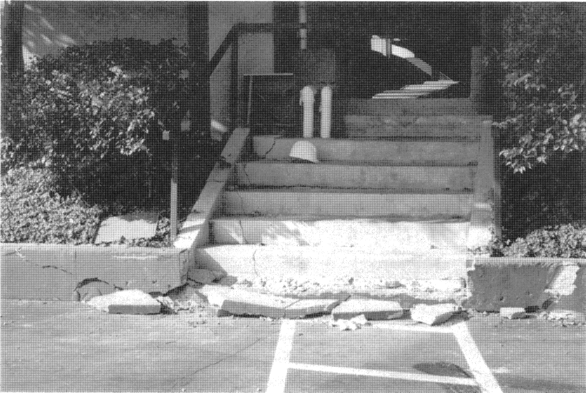
Fig. 4.7: Damage from lateral spreading, Northridge Hospital
