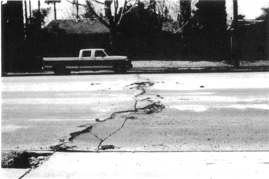
Fig. 4.9: Localized compression feature and pavement damage in Northridge near Highway 118
