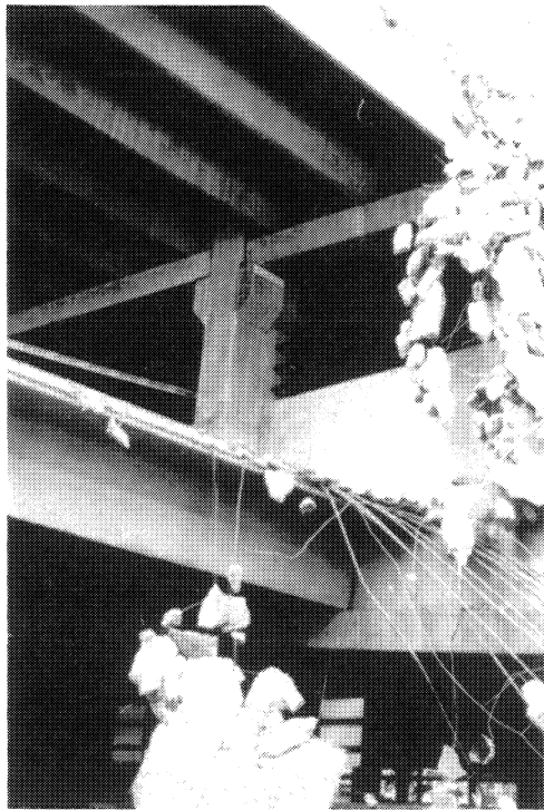
Fig. 6.11 Partial Roof Collapse with Subsequent Punching of Floors Below
